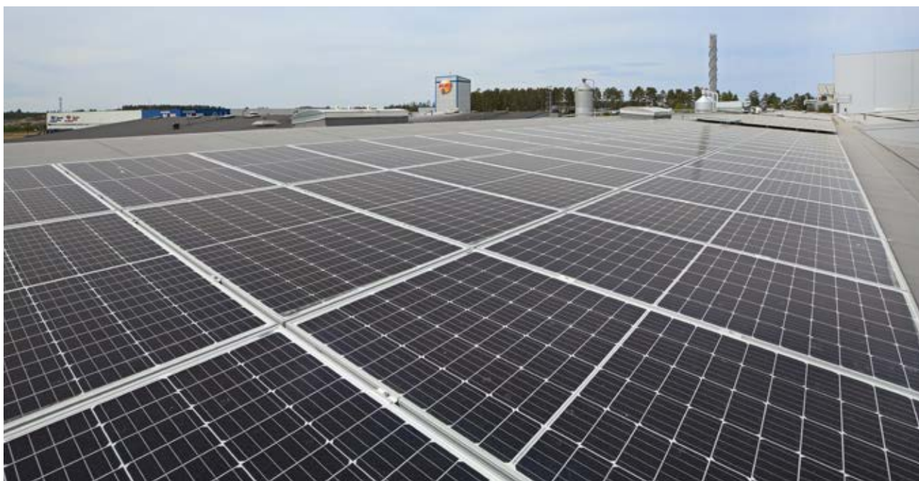
Solar cells on the roof of the property Flahult 21:36 in Jönköping.
