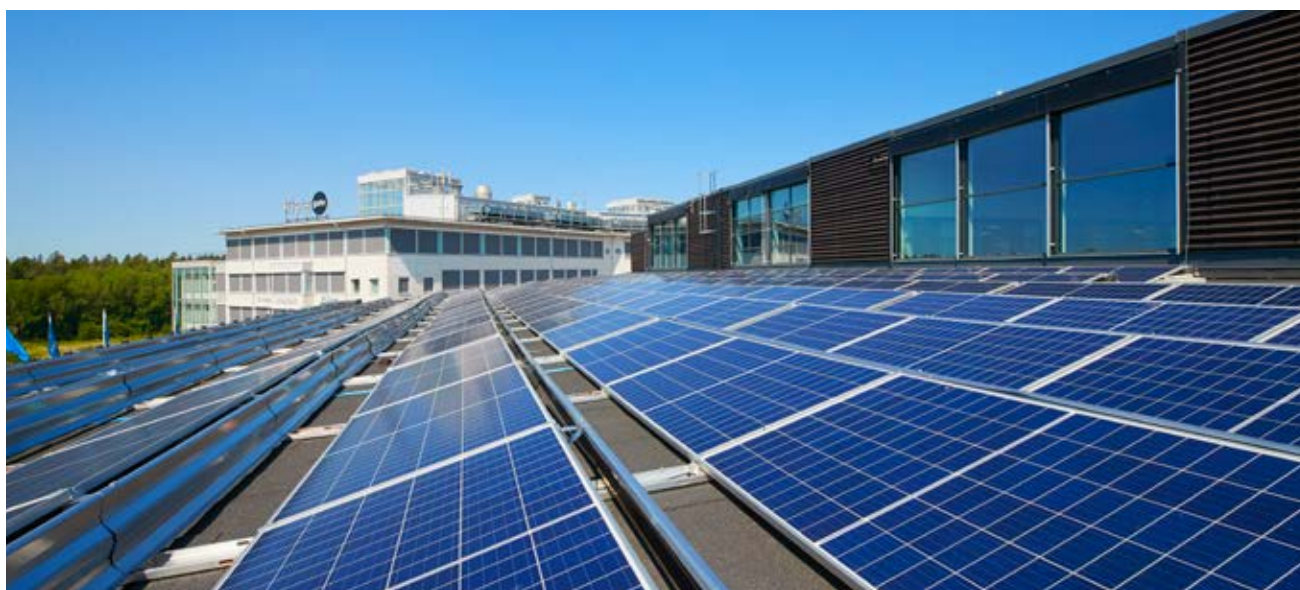
Solar panels on the roof of Kista Gate, Stockholm.
